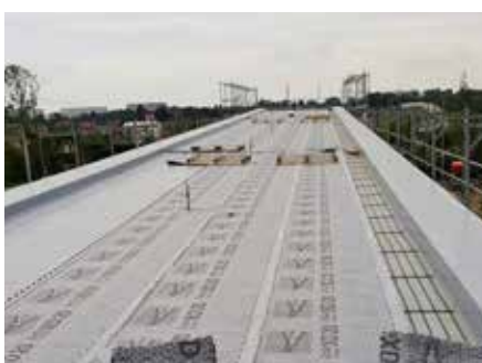
The System Build-up "Rockery Type Plants" provides the foundation, this is the drainage element Fixodrain® XD 20.
